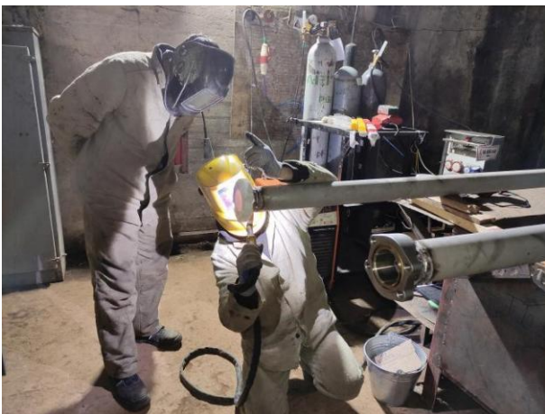
Figure 45. Welding works of the pipe line flanges at the level of 740m (Status in April 2023)
