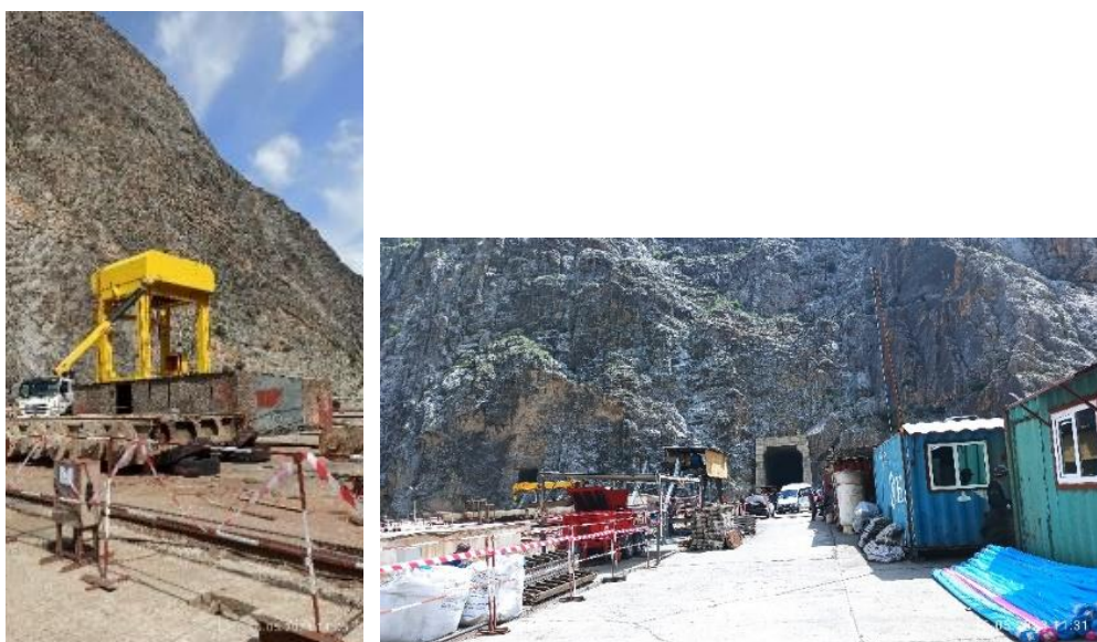
Figure 2. Work areas of CC ZMEC were fenced and clean (Status in May 2023)
