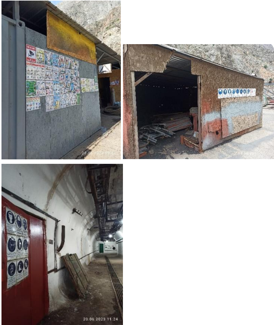
Figure 4. HSE informative signs are placed in all work areas of CC ZMEC (Status in June 2023)
