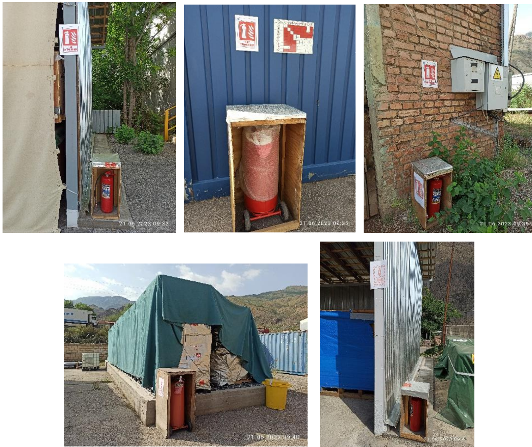
Figure 14. Fire extinguishers installed at CC GE storage site (Status in June 2023)
