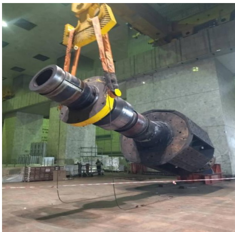
Figure 41. Relocation of disassembled equipment from Unit 2 to the Employer's storage (Status in April 2023).
