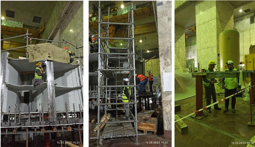
Figure 16. Work staff of CC GE working in compliance with HSE requirements, wearing PPE (Status in May 2023)
