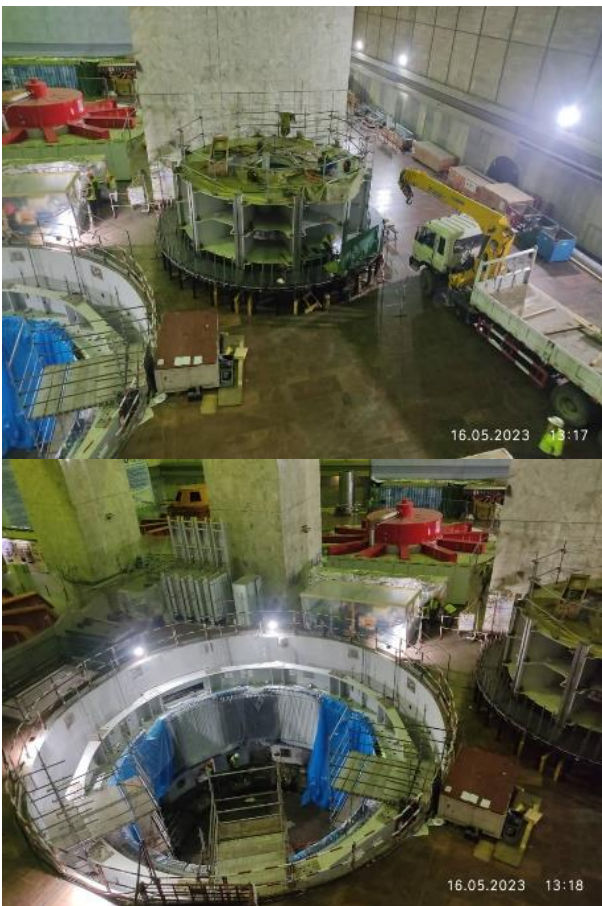
Figure 17. Work area of CC GE in machine hall of Toktogul HPP (Status in May 2023)
