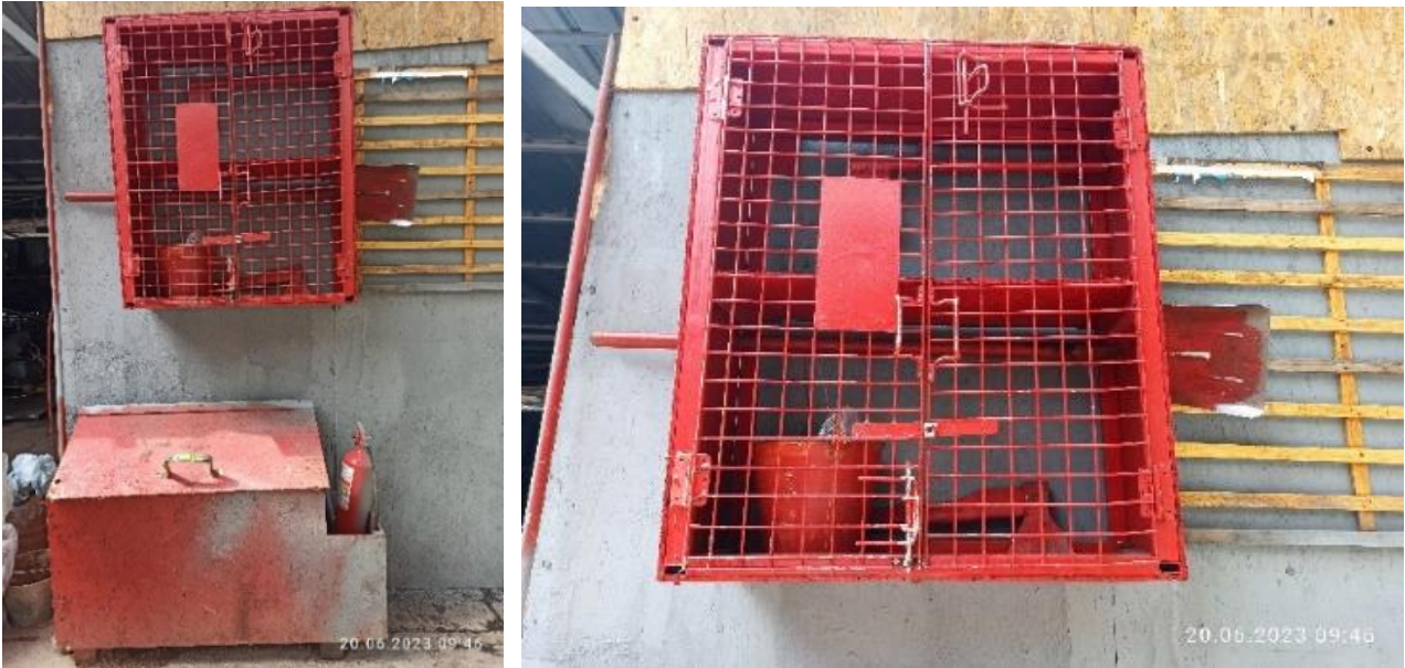
Figure 7. Firefighting equipment of CC ZMEC at site (Status in June 2023)
